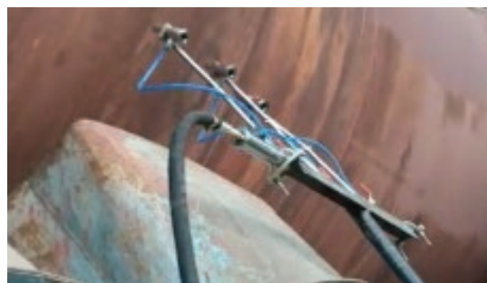
Fig 10: Kiln shell cooling by energy efficient device (Arrest Master ABS)
